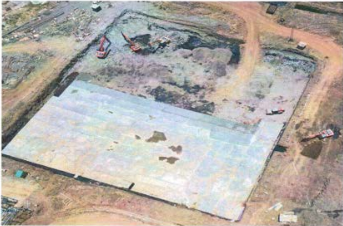
Rainwater/Strom Water Storage Facility
