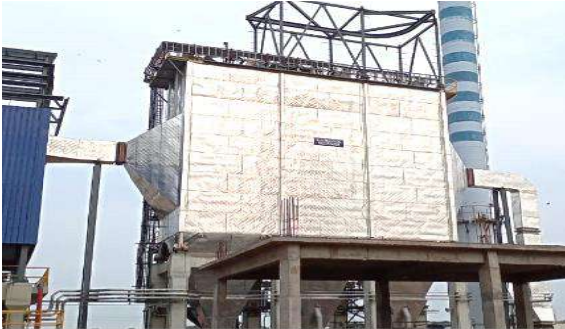
Fig 1. ESP connected to 15 TPH Steam boiler
