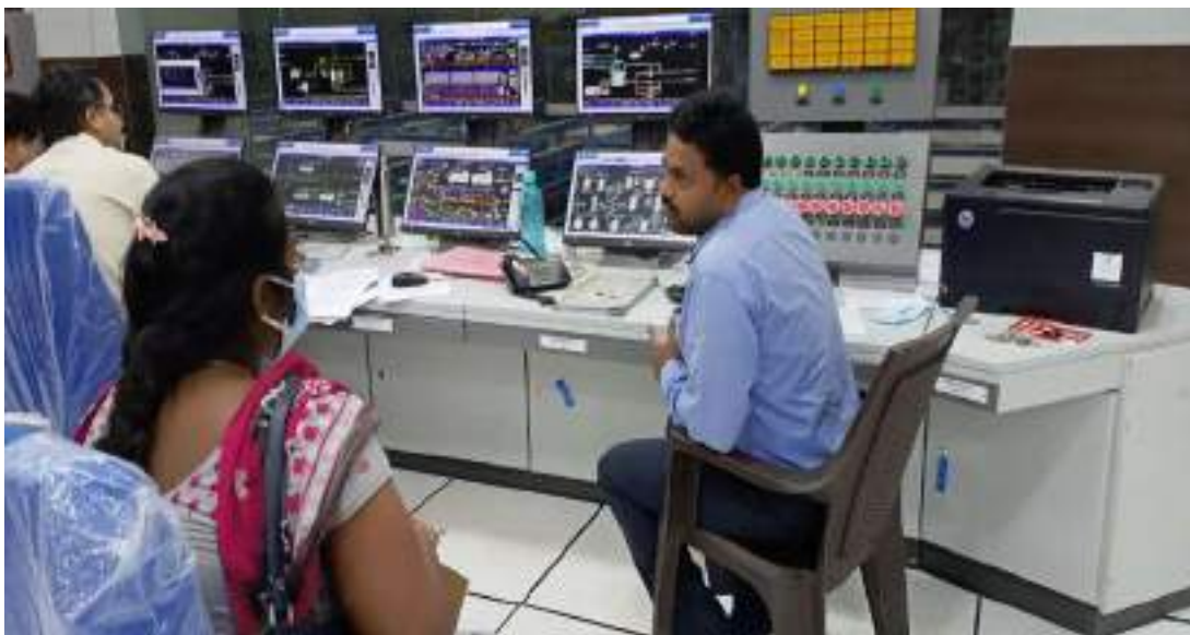
Fig2. DCS control room for carrying out remote operations for entire CAPS (Chlor Alkali products)
