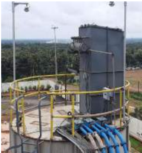
Fig 2. Bag filter installed at Fly Ash Silo
