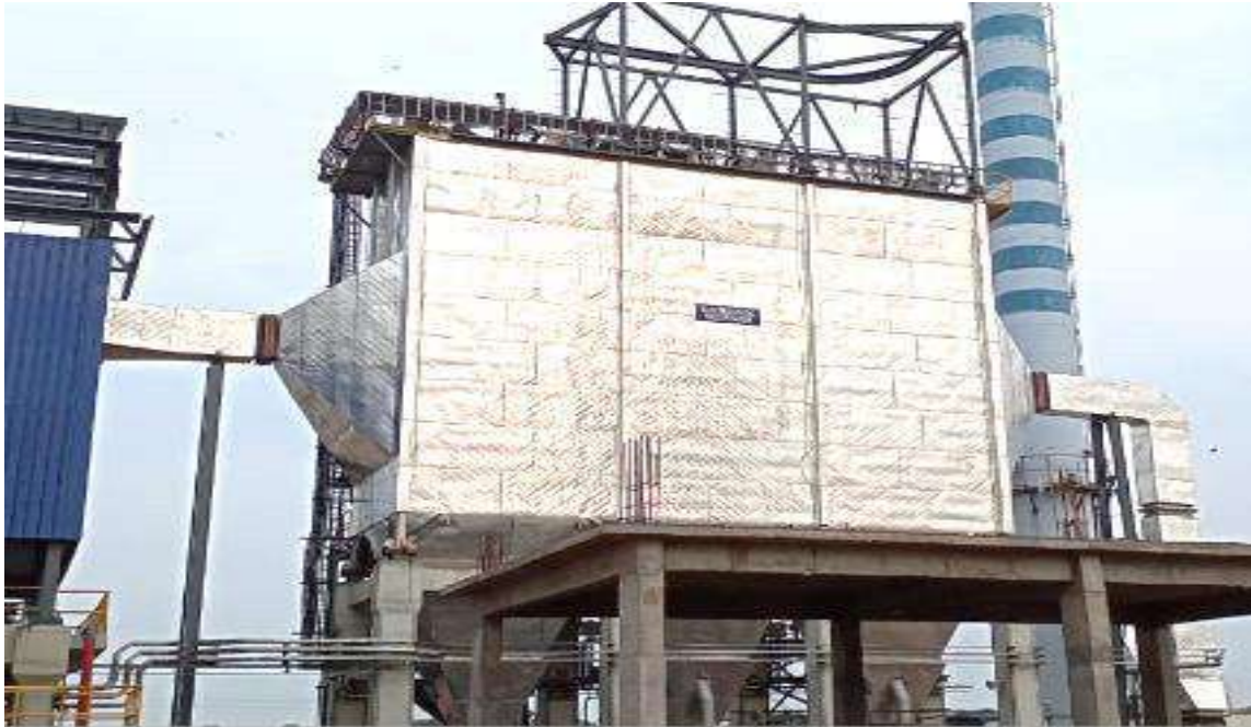
Fig 1. ESP connected to 15 TPH Steam boiler
