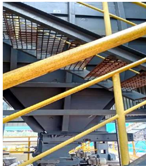
Fig 3. Bag filter installed at Coal transfer tower.
