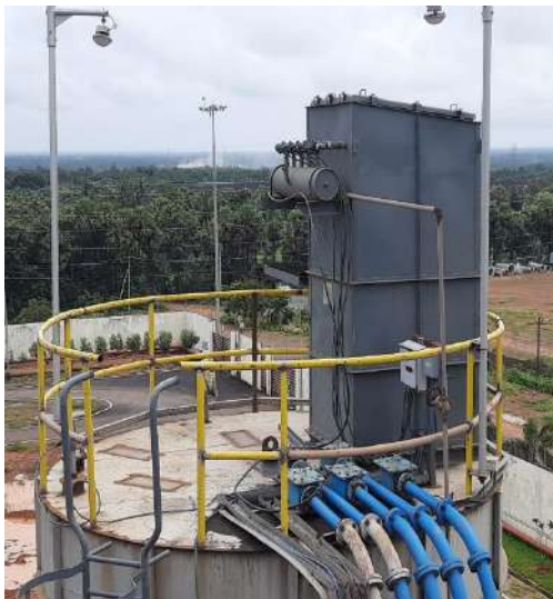
Fig 2. Bag filter installed at Fly Ash Silo
