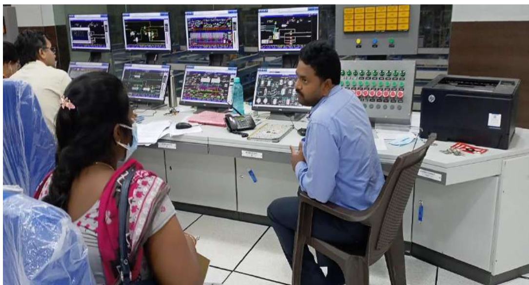
Fig2. DCS control room for carrying out remote operations for entire CAPS (Chlor Alkali products)
