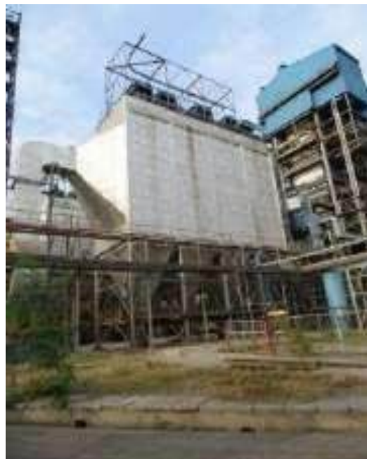
CFBC boiler with 110 m chimney and advanced ESP
