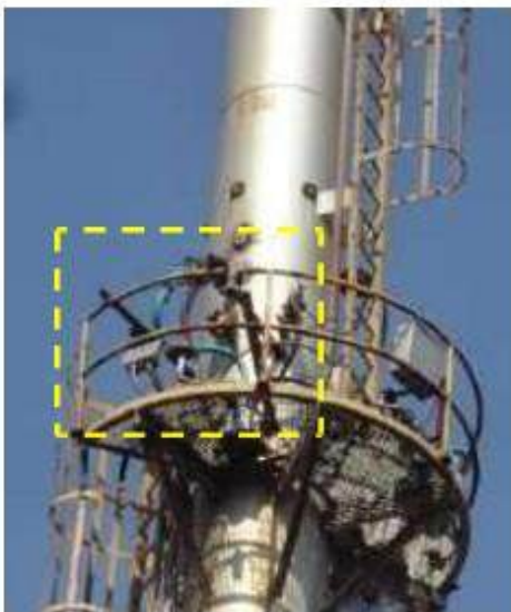
Acid Plant Stack
