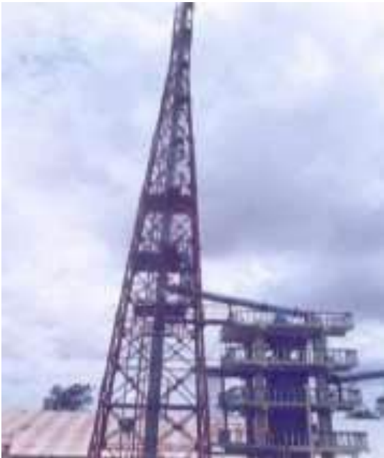
Sulphuric Acid Plant Stack with Alkali Scrubber & Demister to reduce SO 2 emissions and sulphuric acid mist respectively.
