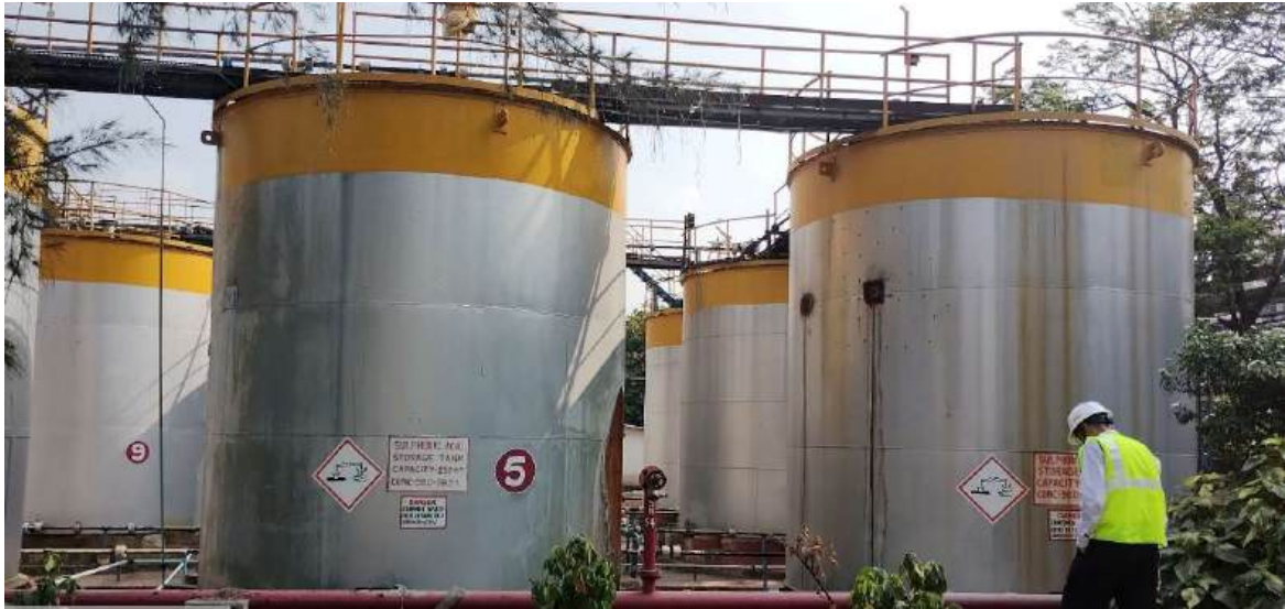
Sulphuric Acid storage tanks
