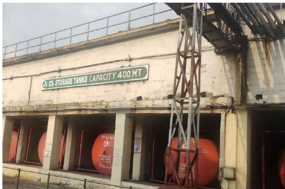
CS 2 Storage Tanks
